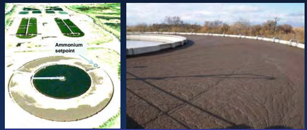
Figure 1. A) Empuriabrava WWTP carousel reactor and reactor with the clarifier in the center; B) Reactor with the clarifier in the center with a foaming episode
