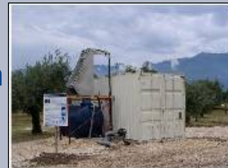
Membrane Bioreactor (MBR)
