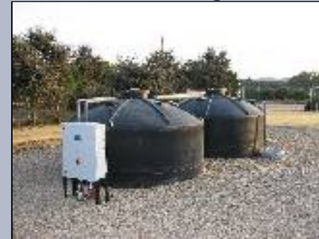
Sequencing Batch Reactor (SBR)
