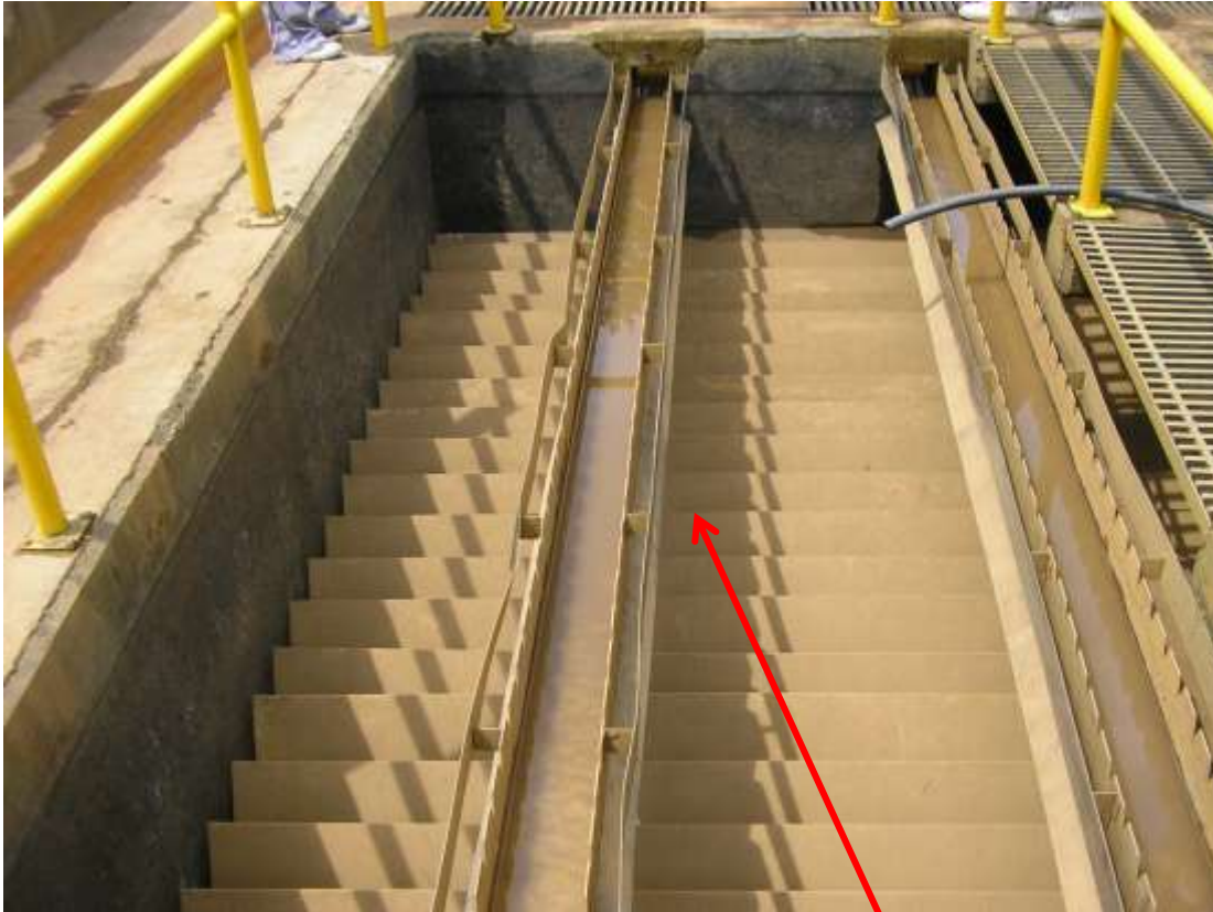
Parallel inclined plate separators
