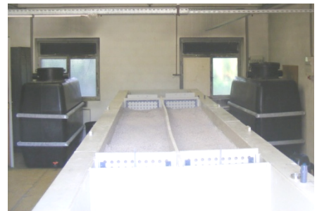
Figure 1 : The two horizontal sand filters
